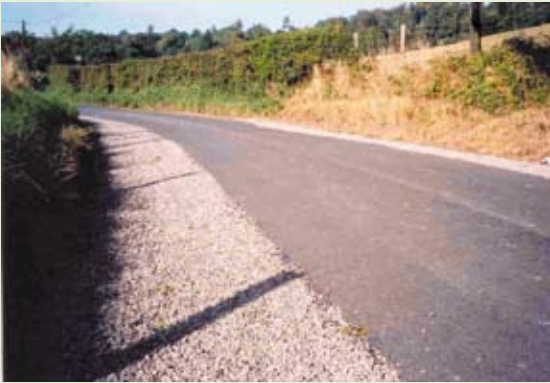
3 Reinforce the 'natural' geometry of country lanes to influence drivers. Surface dressing can be used to visually narrow the road space, help avoid over-running and help create refuge space for other road users.
